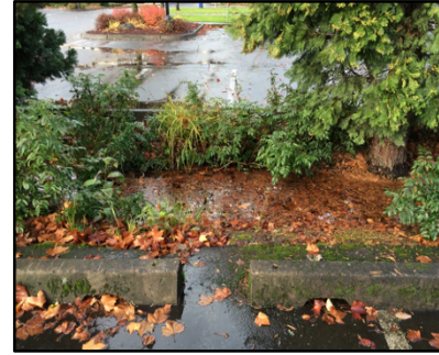
Figure 14: Moto full of stormwater and litter (midway facing west)
