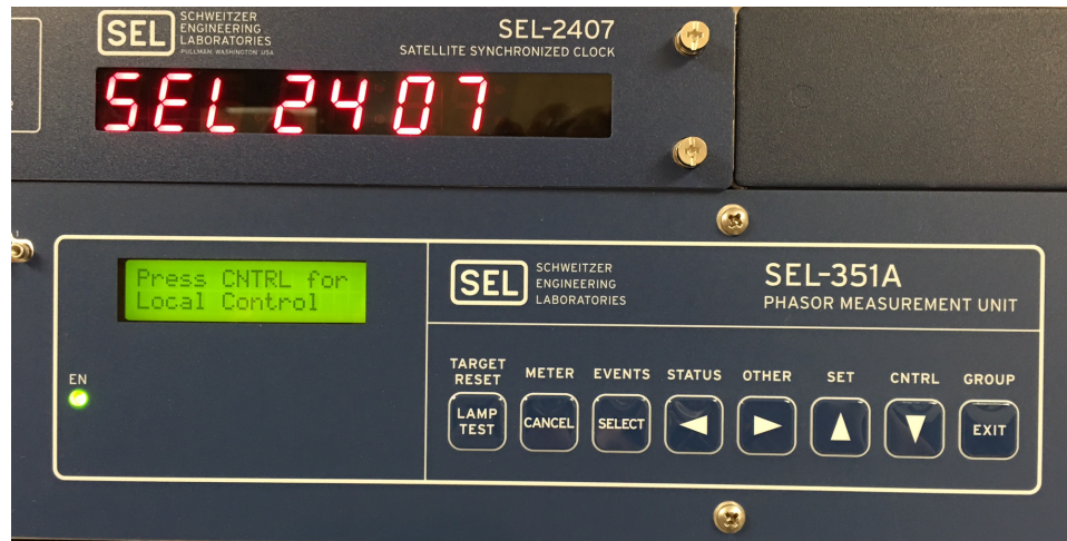
Figure 1.1: Actual Phasor Measurement Unit setup in PGE Power Engineering Lab.
