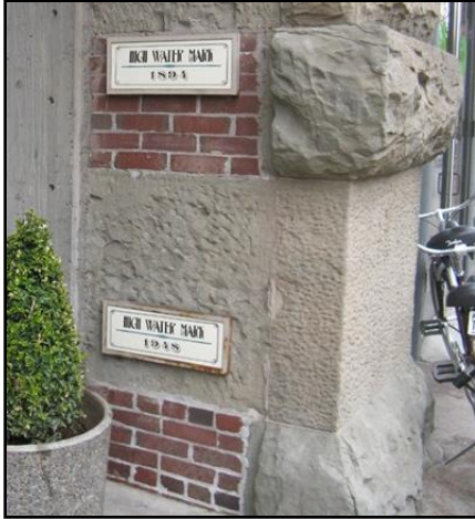
Figure 4-10: Flood marks from the 1894 Spring Flood (top) and the 1948 Vanport Flood (bottom) on the Haseltine building. Photo available at www.waymarking.com
