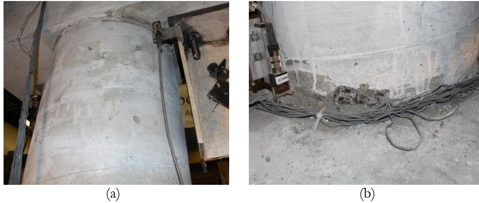
Figure 5.28 Damage in Bent/BRB 2. (a) Horizontal cracks, (b) Spalling of concrete
