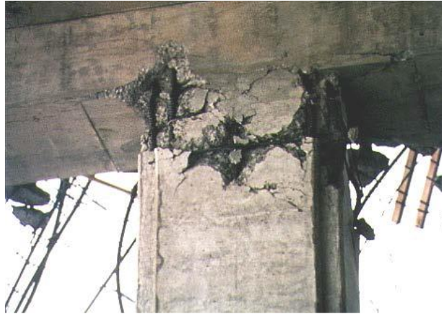
Figure 3.1 Poorly Confined Column in 1971 San Fernando Earthquake
