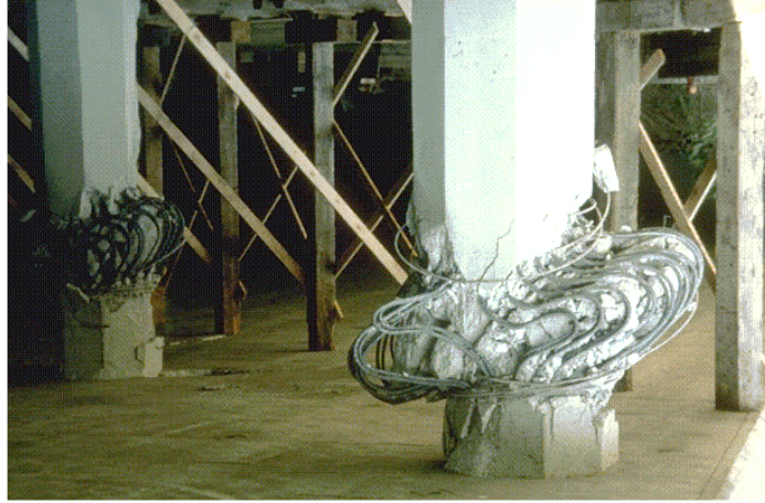
Figure 3.3 Damage in RC columns on the Simi Valley Freeway during the 1994 Northridge Earthquake (Teng, 1994)
