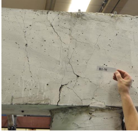
Figure 5.37 Plastic hinge damage in cap beam
