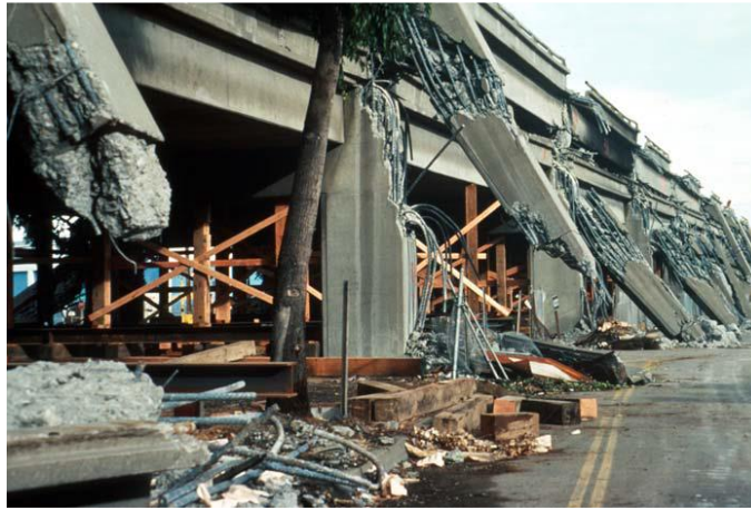
Figure 3.2 Collapsed Cypress street viaduct in Oakland during the 1989 Loma Prieta Earthquake (USGS & Wilshire, 1989)
