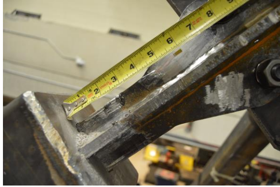
Figure 5.85 Damage in BRB3-Q
