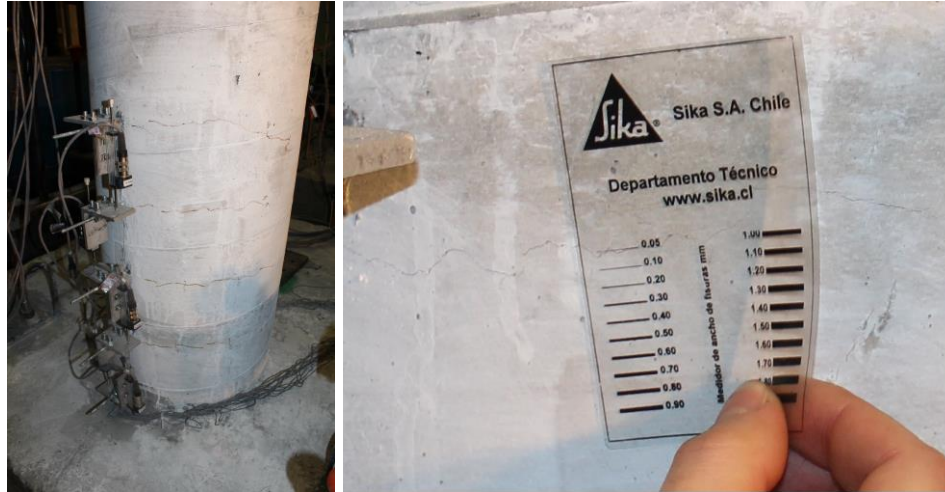
Figure 5.25 Damage in Bent/BRB 1
