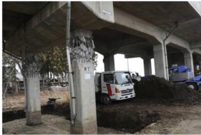
Figure 3.4 Damage in Nakasone viaduct during 2011 Japan earthquake (Kawashima, et al., 2011)
