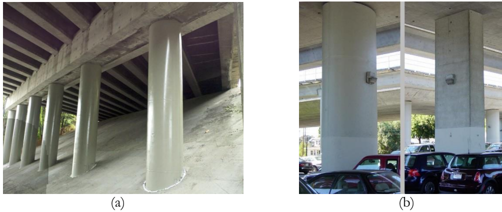
Figure 3.6 Steel Jacketing for: (a) circular bridge columns in Seattle (photo: Lucia Bill), (b) rectangular bridge column in San Francisco. Left: retrofitted column. Right: As-built column (photo, Leonard G.)
