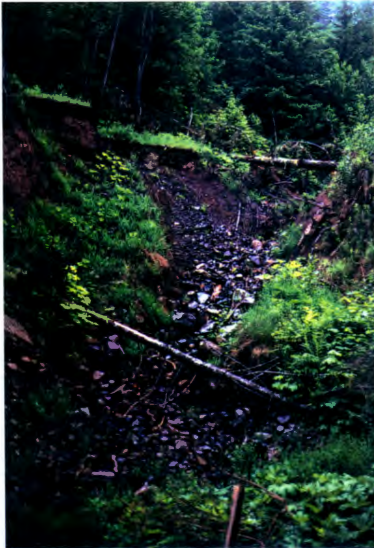
Figure 17. Slump-flow failure in thick glacial deposit - Big Rock Creek, sec. 29, T.5 N. R.5 E. Road failure has occurred where thick till has become oversaturated due to the presence of a perched water table just below the roadbed at the top of the gravel in the left center. The fallen tree at the top of the failure lies in the position of the former roadbed. The stream is flowing from right to left across the bottom of the photo below the green ridge in the foreground, not through the cut below the log.
