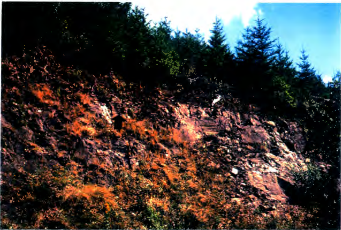
Figure 22. Variation in fracture dilation with depth - FS Rd. 310, NE 1/4 sec. 19, T.5 N. R..5 E. Typical compact igneous bedrock joint dilation habit. Rock mass joints are characteristically platy at the overburden contact (arrow), become more closed and latent with depth and nearly nonexistent furthest away from the contact.
