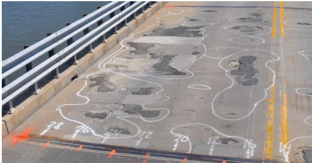
Figure 2-1: Photo of Deteriorated Bridge Deck in Branchport, NJ. Photo Courtesy by Thomas Schumacher.
