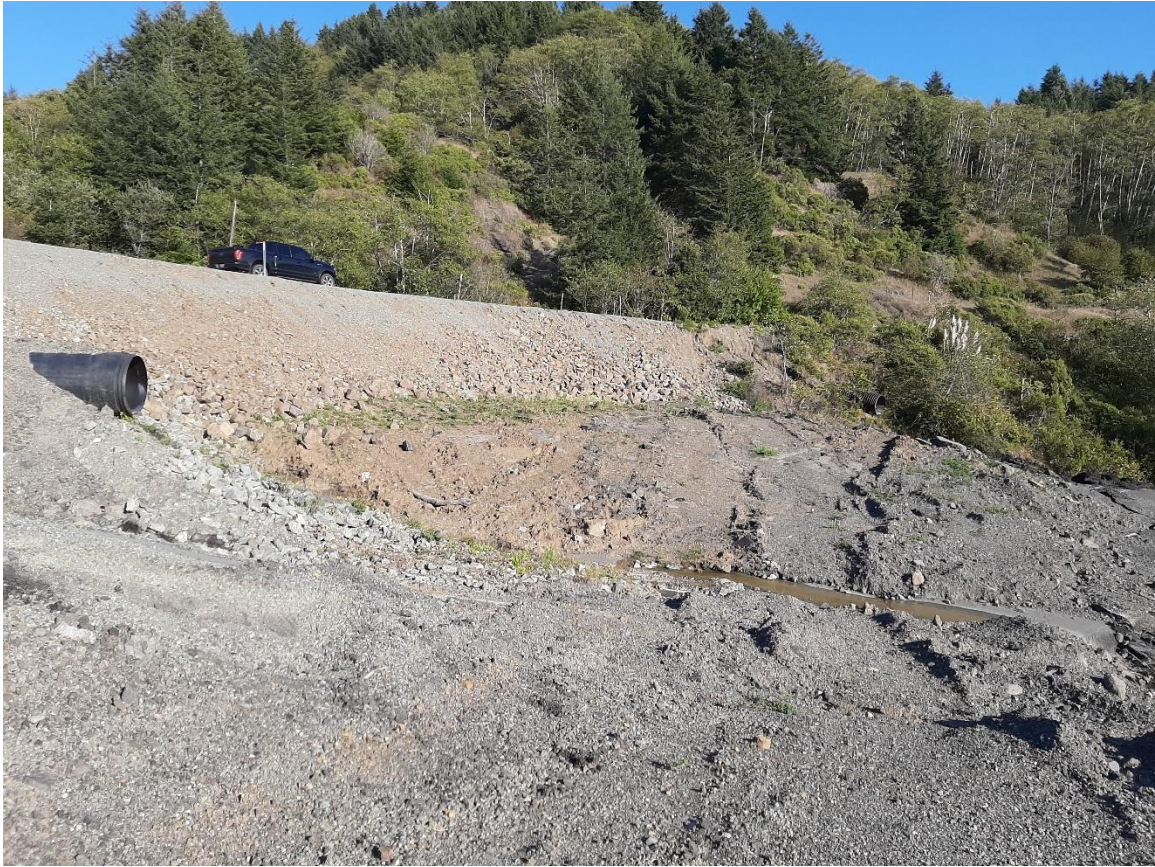
Figure 13: Photograph showing continuous drainage from a culvert installed beneath the newly reconstructed section of US Highway 101, taken in the late summer of 2019.
