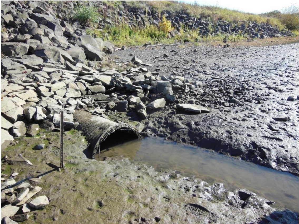
Modern irrigation drainage pipe at site 35MU4.
