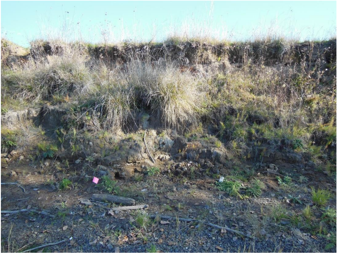
Figure 4.11. Example of severe bank slumping/sloughing at newly identified site PJD002.
