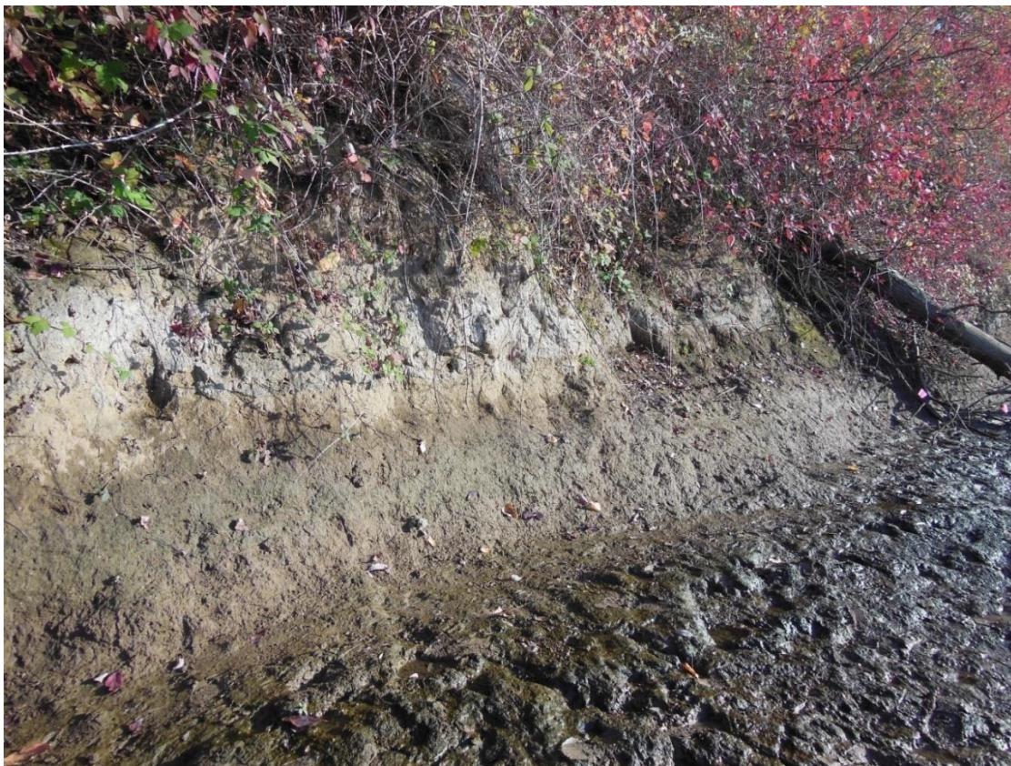
Exposed and high-angled bank at site PJD004.
