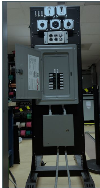
Figure 5.6: This rack provides a power interface between the GS8048A smart inverter and the NHR 9410-12 Grid Simulator.
