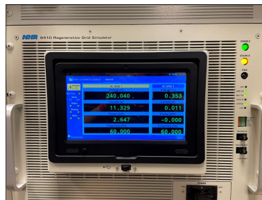
Figure 6.5: Grid simulator export power to load, yellow LED light.
