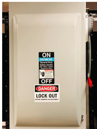
Figure 5.12: Power switch to turn on inverter.
