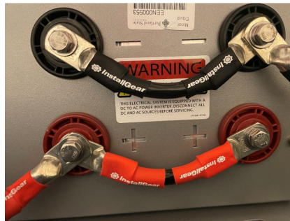
Figure 5.2: Hot and neutral line used to measure battery voltage.
