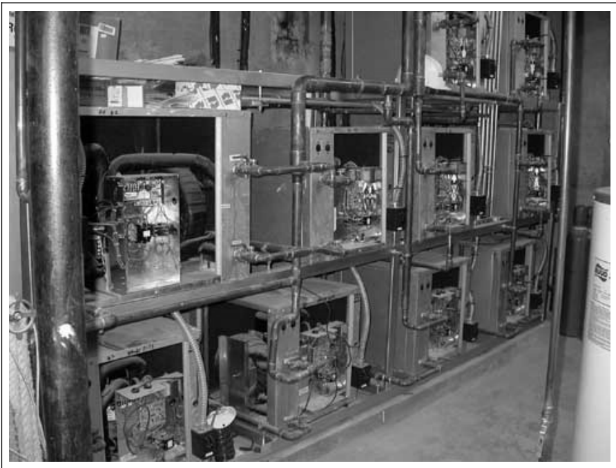
Figure 5. FCNL Building, manifolds for geothermal heating and cooling system
